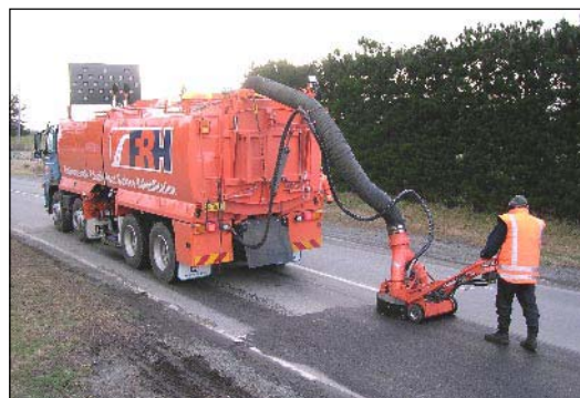
Figure 2 Umbilical Ultra High Pressure Watercutter
