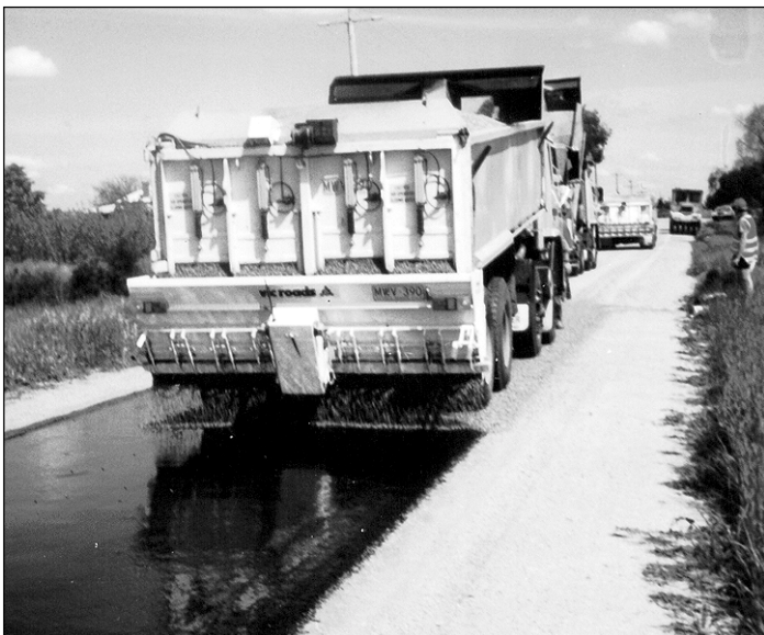
Above: Spreader operated by truck driver; right: spreader operated from a secure platform location
